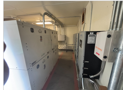
Battery room with CEES™ row and inverter integration
