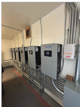
Sol-Ark hybrid inverter array with conduit routing
