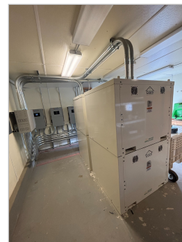
Overhead conduit running from batteries to power conversion system
