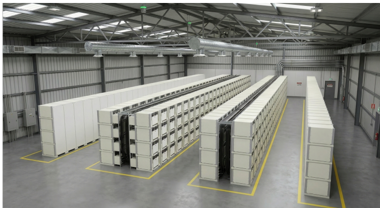
CEES™ BatteryBarn — Multi-megawatt bipolar lead battery installation | Advanced Battery Concepts, Clare, MI
