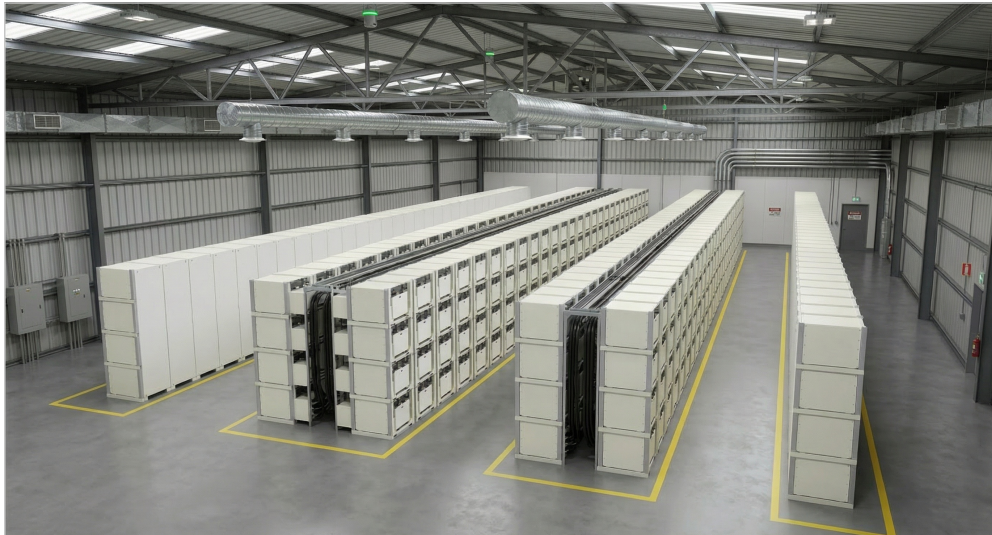
BatteryBarn™: 432 CEES™ cartridges, 4-high by 6-row by 18-column matrix, 20 MWh total capacity
